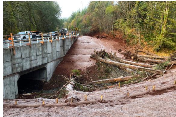
Top: immediately after clear-grub before construction of fish passage structure at Unnamed Tributary to Skookum Creek at MP 5.50 on SR 108. Bottom: completed fish passage crossing, stream channel and slope grading before plantings.
