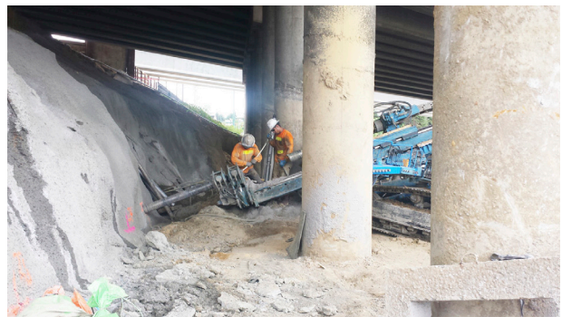
Installation of ground anchors under the existing I-405 bridge at Talbot Road.
