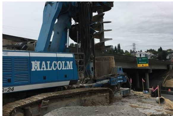
Top: oscillated drilled shafts being installed for the SR167 DC Flyover Bridge. Bottom: construction at the Talbot Road bridge widening.
