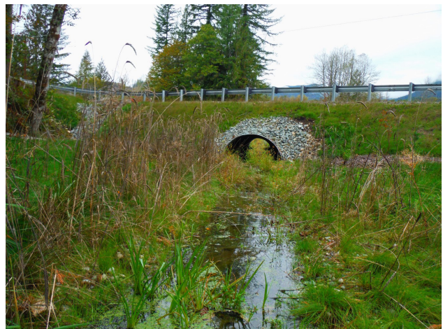
Fully functioning road and fish passable crossing on SR 530 one year after emergency repairs following the Oso landslide.
