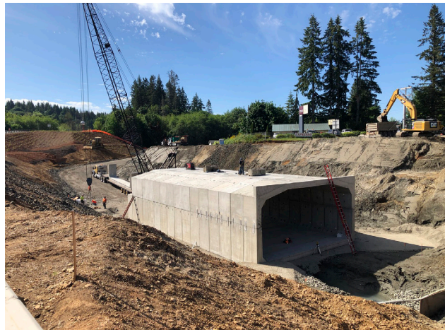
Bottom: fish passage crossing structure installation on a thin, leveling crushed surfacing base course (CSBC), overlaying quarry spalls and geotextile fabric base.
