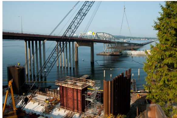
Construction of Pier 2 of the East Approach Bridge on a spread footing.
