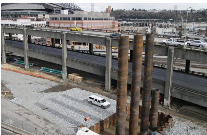
The purpose of the test pile program was to confirm pile capacities and check that vibrations caused by pile driving were below target levels for the nearby active SR 99.
