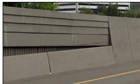
Photo B: Need for Mitigation - Single Slope Barrier Connecting to Tall Wall
