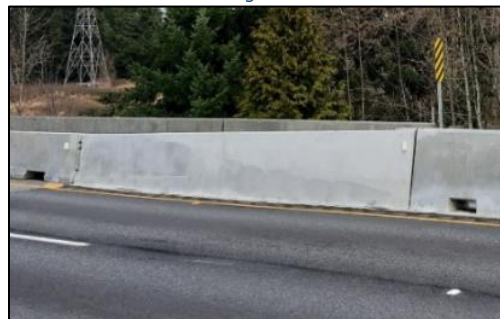
Photo D: Mitigation Strategy - Type F to Single Slope Transition (Height & Shape)
