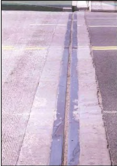
Figure 147. Joint partially filled with debris.
