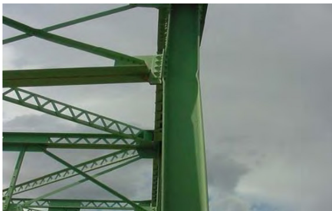
Figure 135. Distortion in truss vertical. Location 1. (Source: Colorado DOT)
