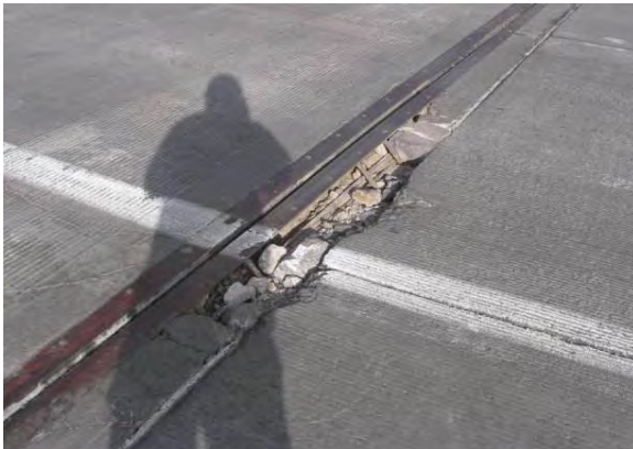
Figure 148. Spall in joint header. (Source: Colorado DOT)
