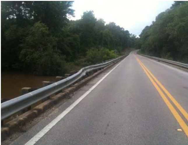
Figure 143. Collision-induced distortion of bridge railing.
