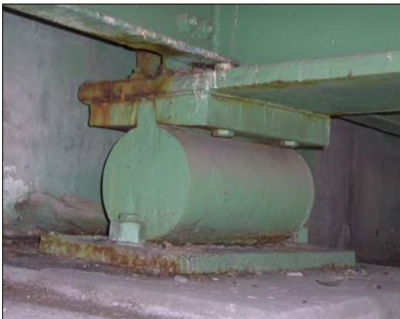
Figure 146. Surface rust on moveable bearing.
