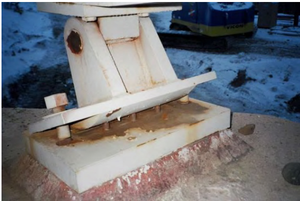
Figure 145. Misaligned rocker bearing. (Source: Alaska DOT)
