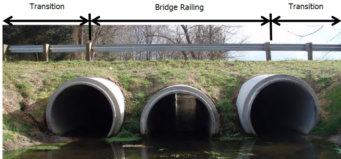
Figure 12. Metal bridge railing and transition for long-span application. (Image Source: Delaware DOT)
