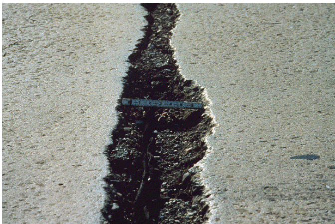
Figure 132. Deck spalling along joint. Location 2.
