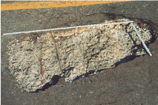
Figure 133. Typical deck spall with exposed rebar. Locations 3 and 4.
