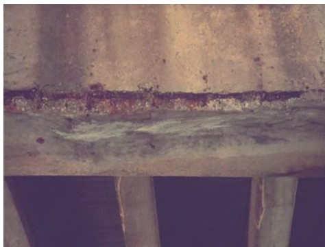
Figure 138. Spall in Pier 2 cap beam. Location 1.
