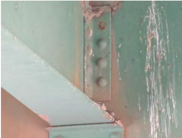
Figure 136. Missing rivets in stringer-to-floor-beam connection. Location 4. (Source: Colorado DOT)
