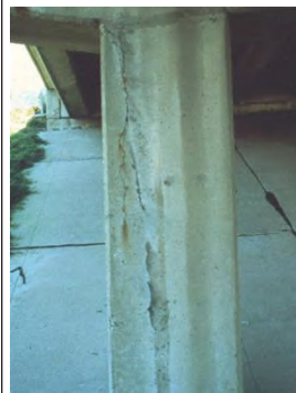
Figure 139. Crack in Pier 3 column. Location 3.
