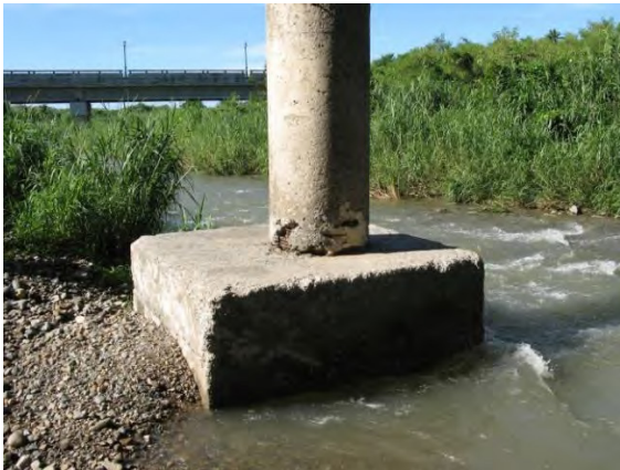
Figure 153. Exposed column footing in stream.
