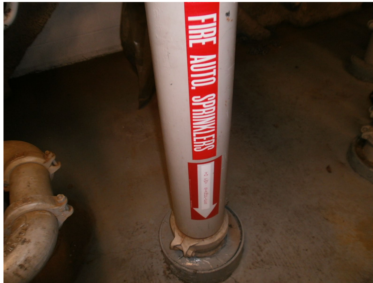
Photo 2 Standpipe Labels – non-compliant with ANSI/ASME A13.1
