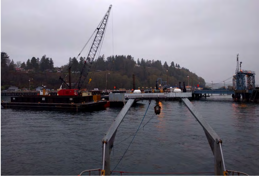
Figure 2a. Photograph from the stern of the anchored R/V Robertson overlooking the A-frame and looking toward the construction barge complex, taken at 9:00 am on 7 December.
