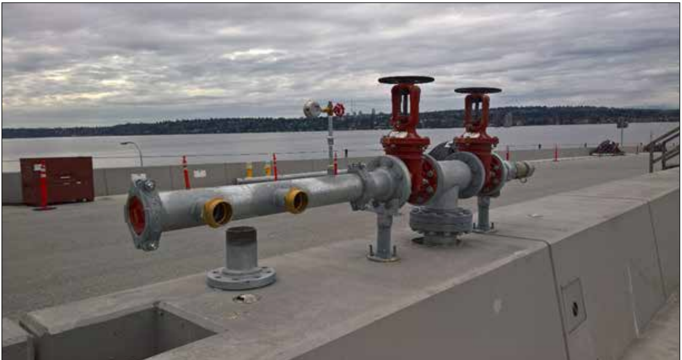
Fire safety systems: Pipes, hydrants and pumps installed for the fire safety system provide firefighters with water to extinguish a fire if one should occur on the bridge.
