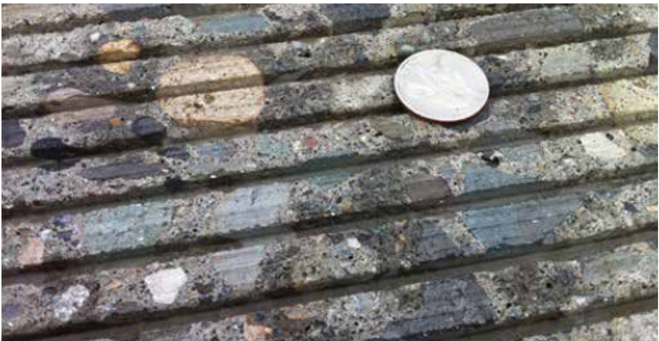
Roadway grinding: The 34,580 square feet of roadway on the floating bridge features Next Generation Concrete Surface grind – grooves in the pavement to reduce traffic noise. Learn more about quieter concrete research in Washington state at www.wsdot.wa.gov/Business/MaterialsLab/QuieterPavement/
