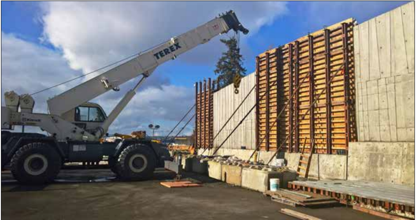
Noise walls: To minimize traffic noise in nearby areas, crews constructed 1,600 feet of noise walls along the north and south sides of the bridge in Medina.
