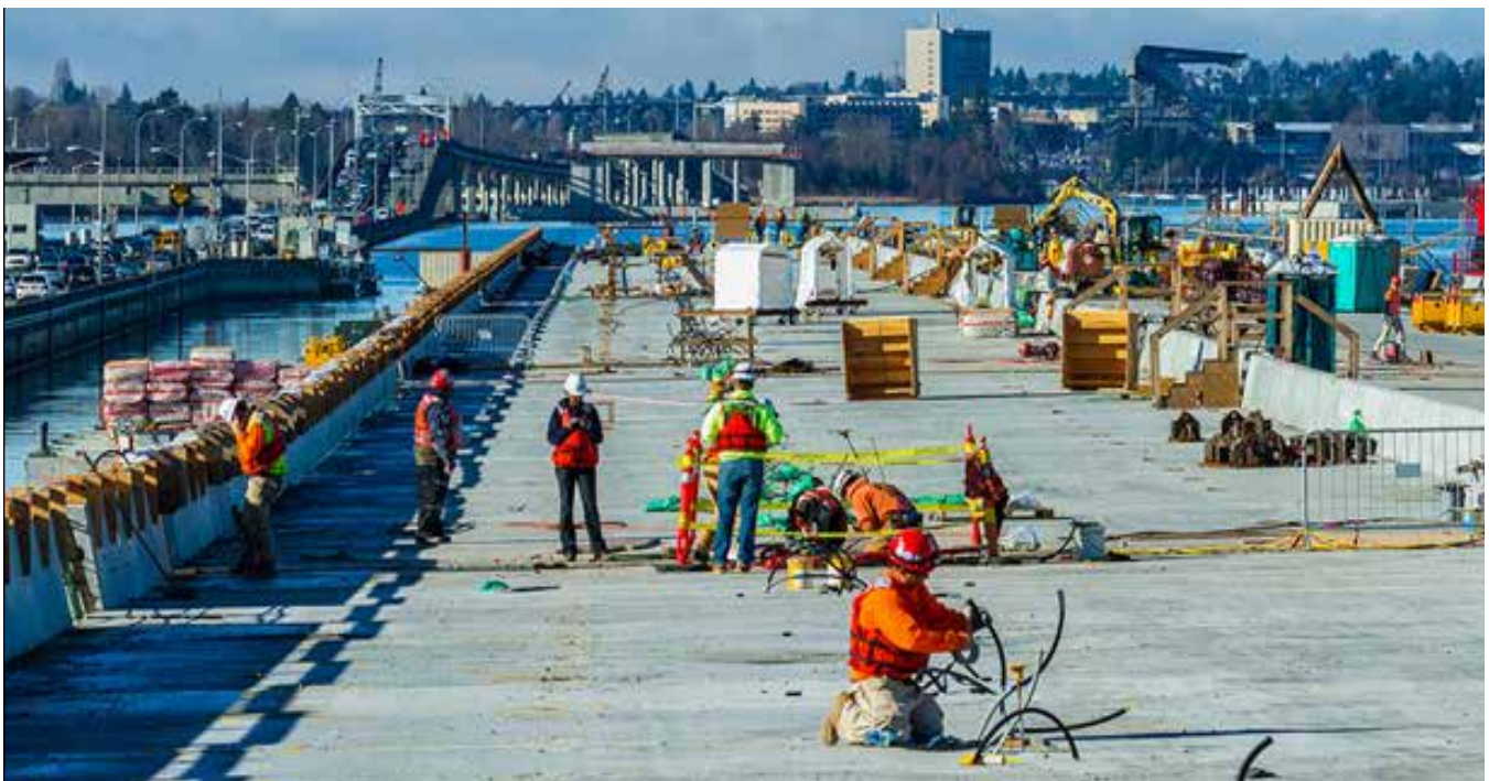
Bridge barrier: There are 25,846 feet of barrier installed along the length of the bridge. The barriers separate the highway's eastbound and westbound lanes, as well as the new regional shared-use path.
