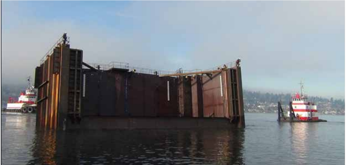
This coffer cell was used to make in-water repairs of two Cycle 1 pontoons.
