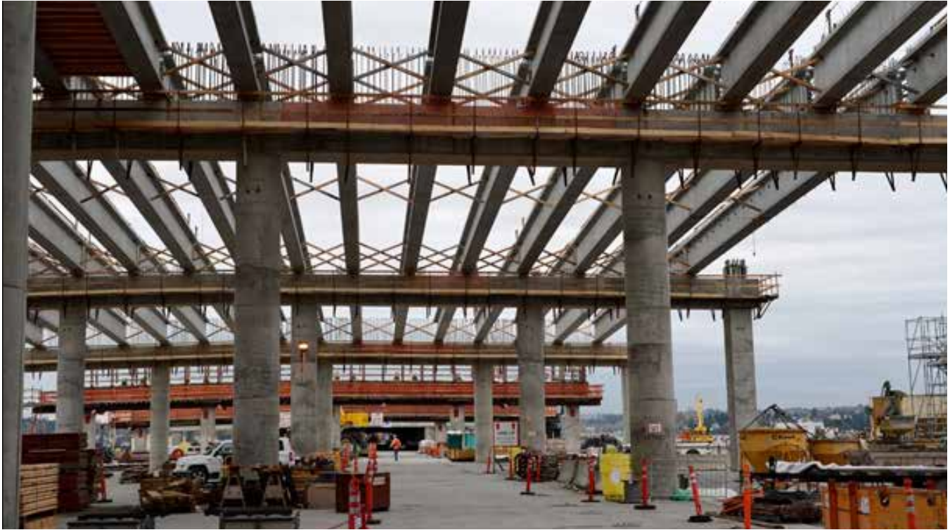
Deck support: The bridge deck is supported by 771 concrete columns and 331 concrete girders, large beams that the bridge deck rests upon.
