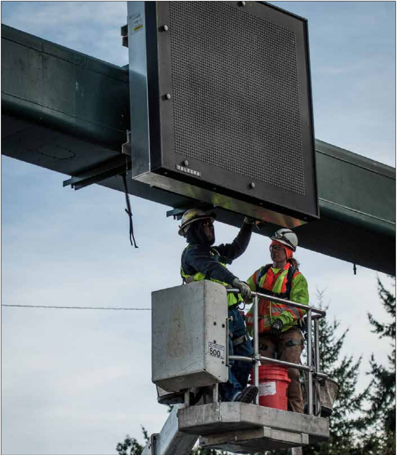
Static and active traffic management systems: Modern traffic signage and electronic speed-limit notifications keep traffic flowing, with 105 new traffic signs and gantries installed.
