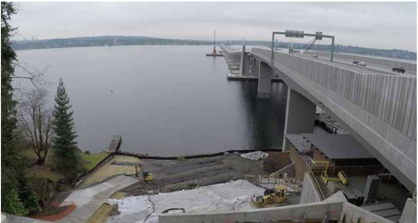
Medina viewpoint: One of the final tasks on the Floating Bridge and Landings Project is construction of a pedestrian trail and lakeside viewpoint in Medina. Shown here is the viewpoint construction site just south of the bridge.
