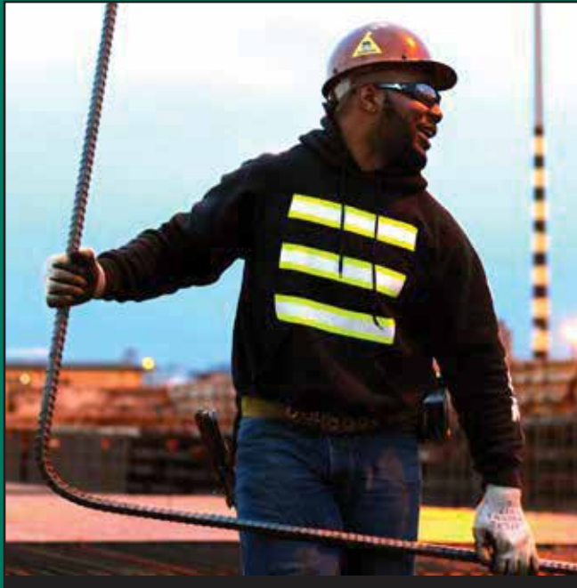
An ironworker lifts rebar at the pontoon casting basin in Tacoma, January 2013
