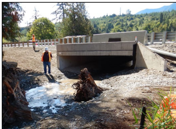
Figure 47. The new crossing is an 18.2 ft span by 10 ft rise concrete box culvert that allows passage for chum, coho, steelhead, coastal and resident cutthroat trout.
