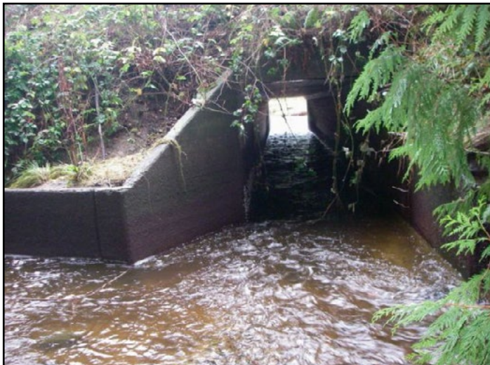
Figure 35. The old crossing was a 6 ft square concrete culvert that was a depth and velocity barrier during low tide.
