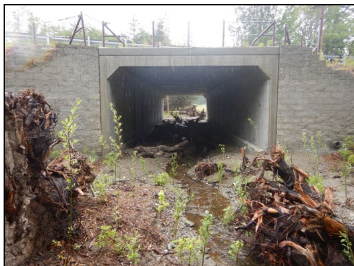
Figure 43. The new crossing is a concrete culvert with an 18.27 ft span, 19 ft rise, and is 80.16 ft long. Wildlife connectivity safety factors ranked high at this site, justifying the addition of wildlife benches up to 5-10 ft wide were constructed above the 2-year flood elevation.
