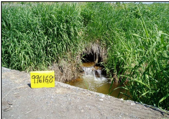
Figure 9. This culvert was 2 ft in diameter, round, and made of mixed materials with a corrugated steel inlet and cast concrete outlet.
