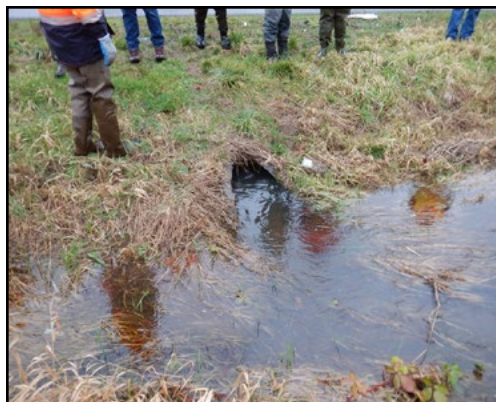
Bottom (990688): Old crossing was a 2 ft diameter culvert measuring 78 ft long and was a velocity barrier.
