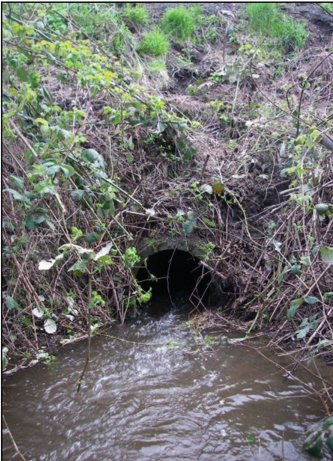
Figure 44. The old crossing was a 2 ft diameter concrete culvert that was a barrier due to slope.
