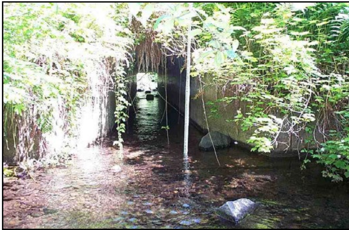
Figure 31. The old crossing was a 6.1 ft square cast-in-place concrete culvert that was both a velocity and depth barrier.
