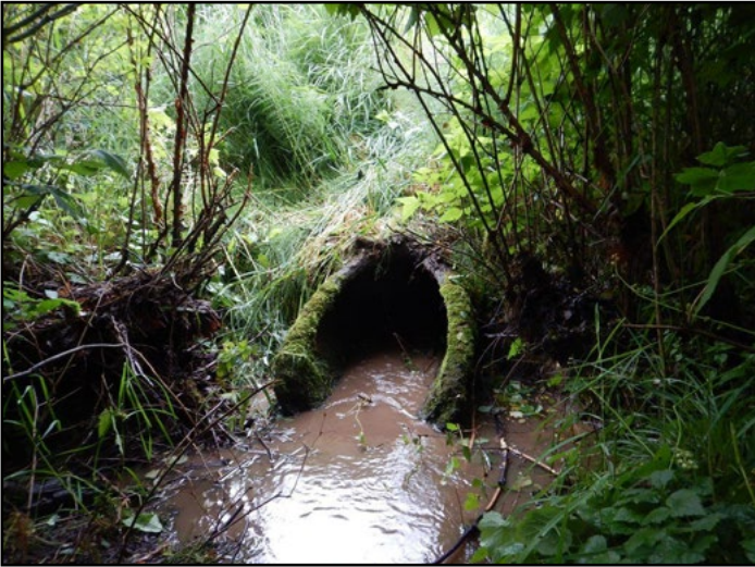
Figure 48. The old crossing was a 2.5 ft diameter concrete culvert that was a barrier due to slope.
