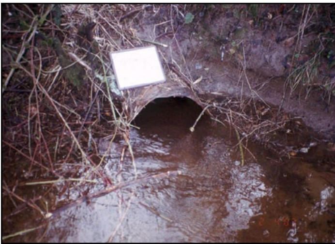
Figure 19. The old 2 ft diameter culvert consisted of mixed materials, with a corrugated steel outlet and a concrete inlet.
