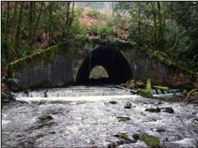
Figure 53. The old crossing was a concrete arch-shaped culvert retrofitted with a fishway. The dimensions were 19.5 ft span by 15 ft rise and 210 ft long. The fishway consisted of baffles composed of a series of jersey curbs strapped and bolted end to end spaced every 10 ft through the length of the culvert with weirs on the culvert aprons. The fishway was assessed as a barrier due to excessive hydraulic drop over the weirs.
