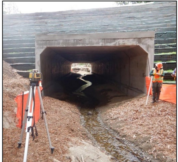
Figure 40. The new crossing is a concrete bottomless arch culvert with a 17.5 ft span, 17.0 ft rise and is 130 ft long.
