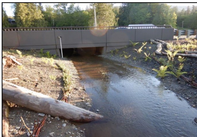
Figure 12. The new structure is a concrete box culvert 11.2 ft span and a rise of 8.0 ft. The new structure improved access to 1.0 mile of potential habitat.
