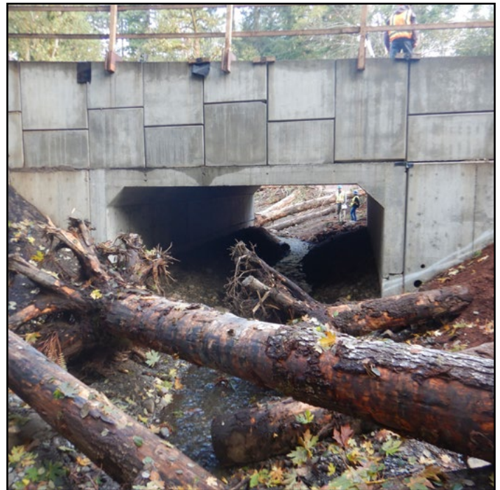
Figure 30. The new crossing is an 18 ft span by 13.7 ft rise concrete box culvert.
