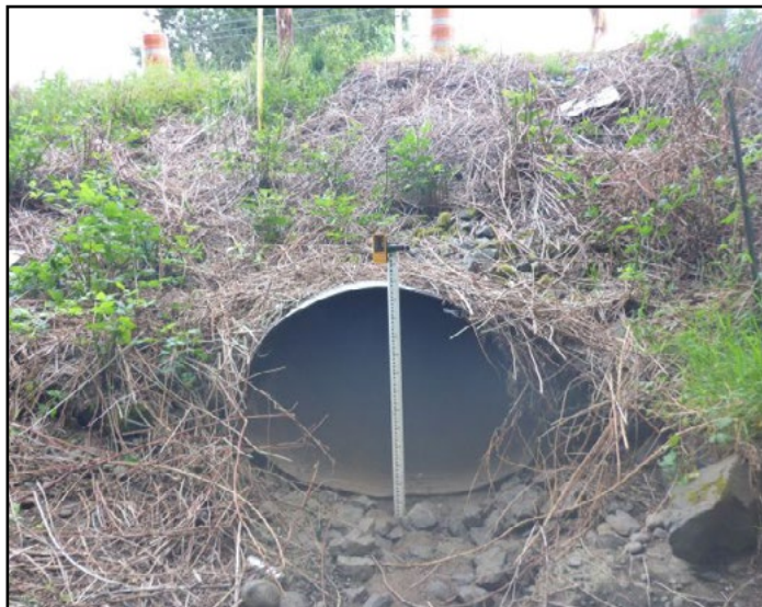
Figure 21. The old crossing was a squash, corrugated steel culvert with a 5.9 ft span and 3.8 ft rise. It was a partial barrier to fish passage due to shallow water depth and debris accumulation.
