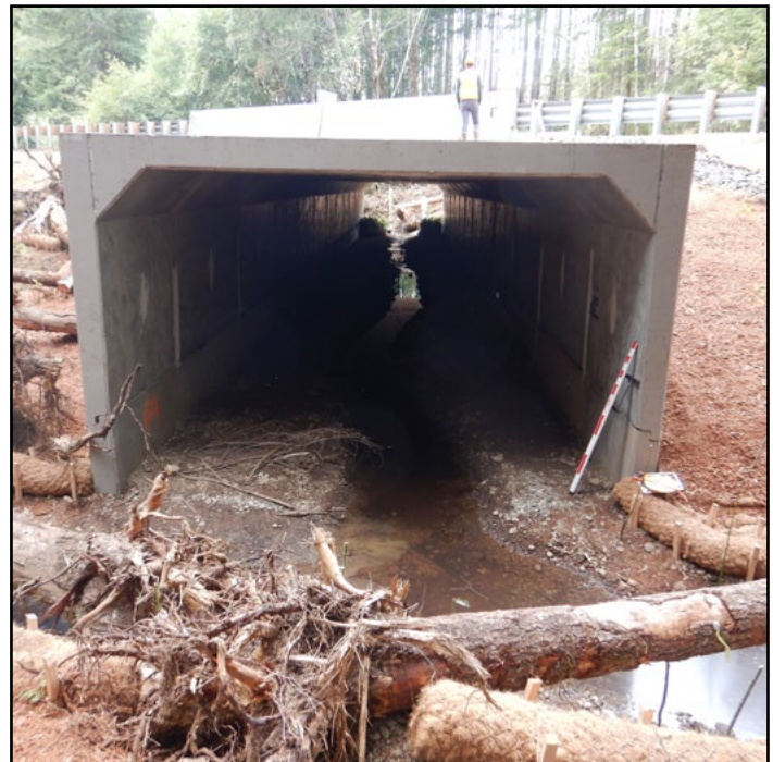
Figure 60. The new crossing is a 15.1 ft span by 14.1 ft rise concrete box culvert.
