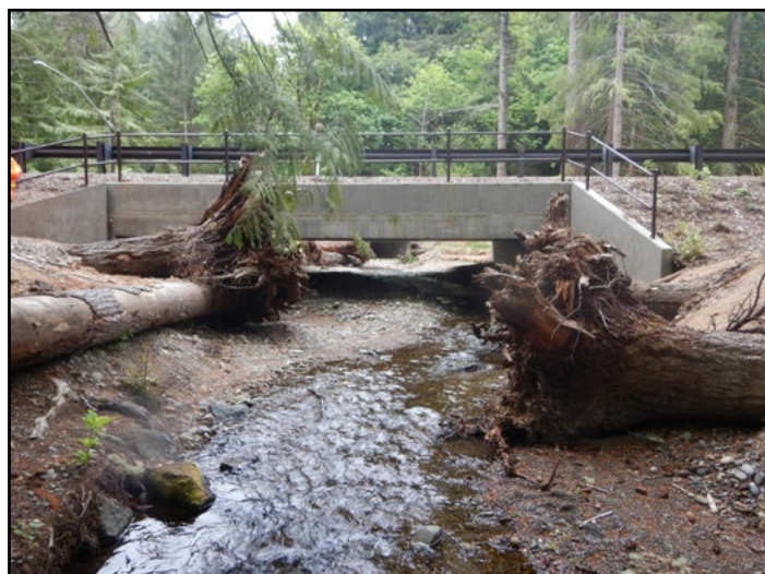
Figure 28. The new crossing is a 29.2 ft span by 7 ft rise concrete box culvert.
