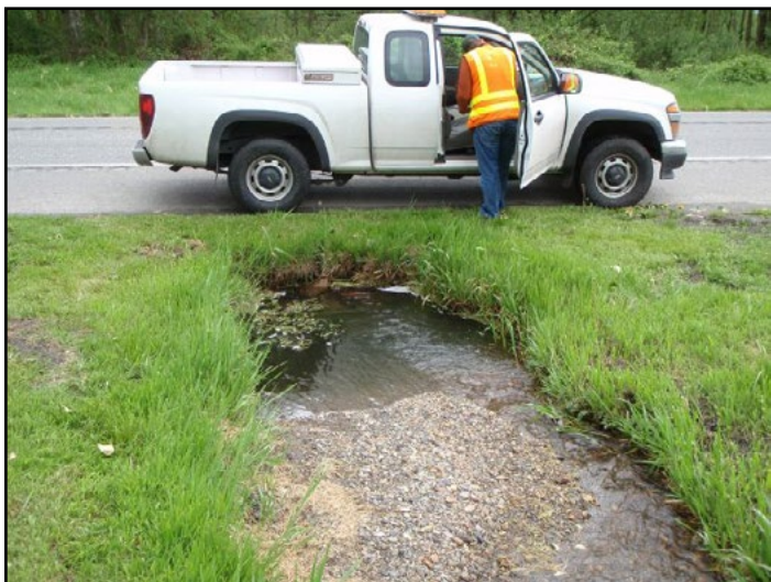
Figure 11. The old crossing was a concrete, round culvert with a diameter of 1.5 ft and 50.5 ft long. The structure was considered a velocity barrier due to excessive culvert slope.
