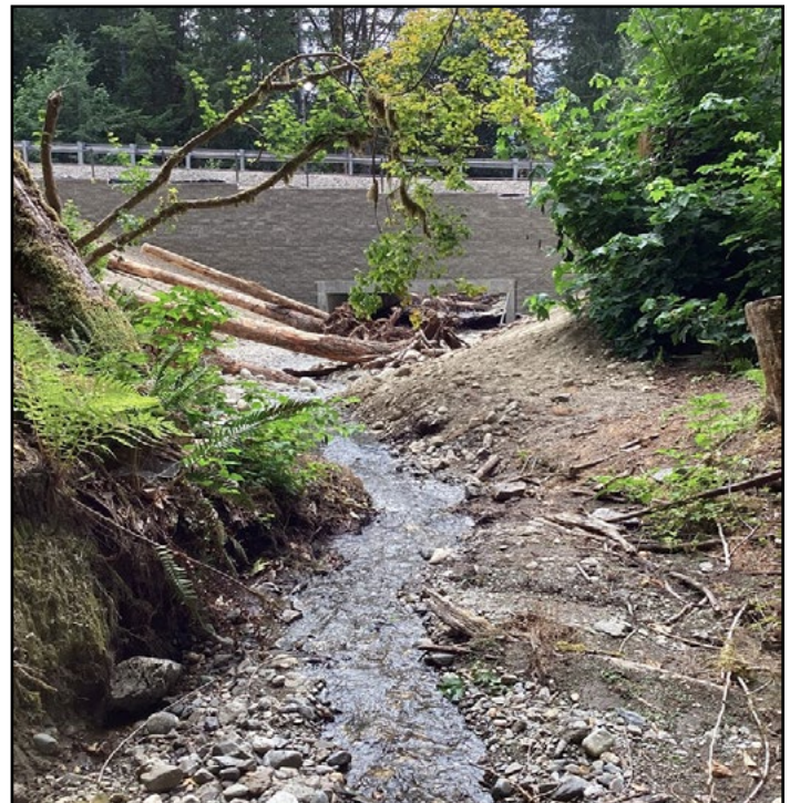
Figure 16. The new structure is a concrete bottomless culvert with a 19.8 ft span, 15 ft rise, and is 55 ft long.
