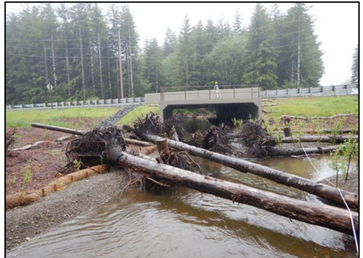
Figure 62. The new crossing is a 25.3 ft span by 12 ft rise concrete box culvert.
