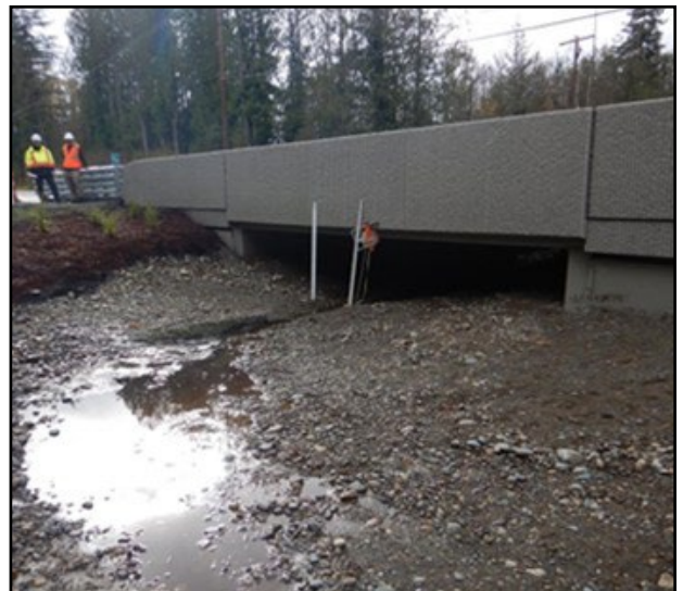
Figure 26. Top (991225): The new concrete box culvert has an 18.2 ft span, 9.4 ft rise, and is 42.6 ft long.
