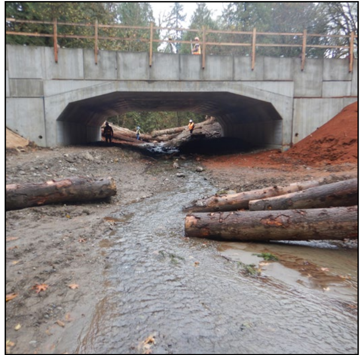
Figure 32. The new crossing is a 35.1 ft span by 16.8 ft rise bottomless arch culvert.
