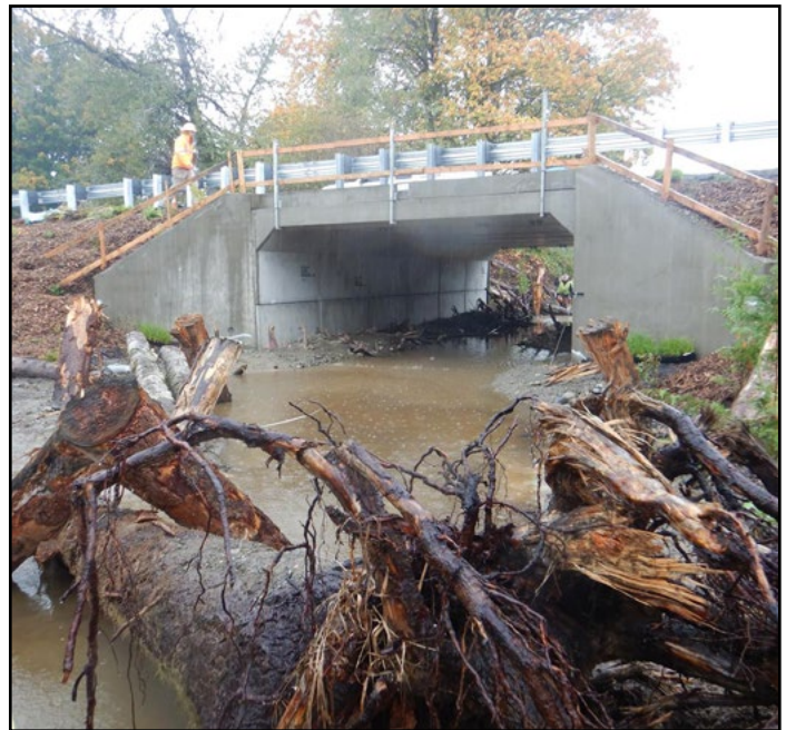
Figure 20. The new crossing is a concrete box culvert with a 19.3 ft span and a 13.7 ft rise.
