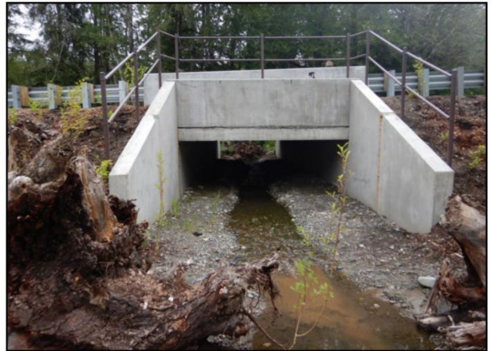
Figure 49. The new crossing is a 13 ft span by 9 ft rise concrete box culvert.
