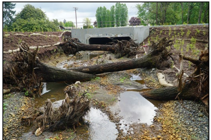
Figure 6. The new crossing was moved to the north and skewed across SR 539 to better align the creek as it crosses to the highway. The new crossing is a concrete box culvert with a 20 ft span, and 12 ft rise. The original two culverts remain in place, one filled/abandoned and the other converted to stormwater conveyance which is managed by the City of Lynden.
