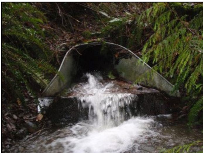
Figure 15. The old crossing was a 2.5 ft diameter corrugated steel culvert with aprons on both ends, measuring 121 ft long. The crossing was assessed as a barrier due to an excessive hydraulic drop at the outlet.
