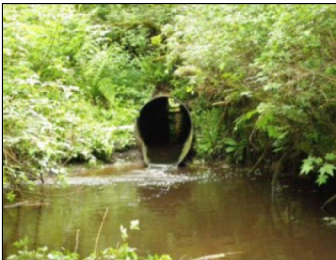
Figure 39. The old crossing was a 163 ft long, 4.75 ft diameter corrugated steel culvert assessed as a barrier due to excessive velocity.
