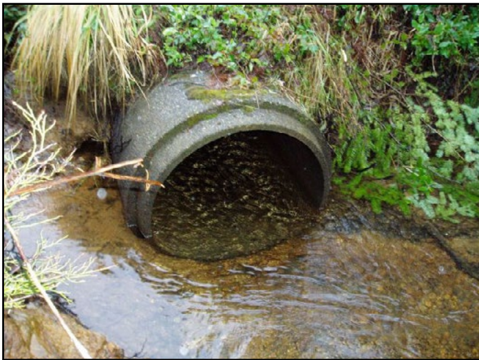
Figure 59. The old crossing was a 3 ft diameter concrete culvert that was a slope barrier.
