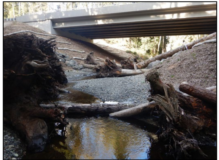
Figure 38. The new crossing is a 110 ft concrete girder bridge. Due to the proximity to public lands, open space, and high wildlife vehicle collision areas, the new crossing was designed with wildlife benches to accommodate deer passage beneath the new bridge.
