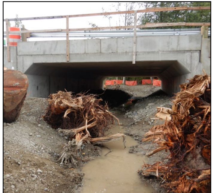
Figure 45. The new crossing is a 20 ft span by 11.5 ft rise concrete bottomless arch culvert. To accommodate potential use by amphibian species in a nearby wetland and proximity to state-endangered fisher distribution range, the structure provides a wildlife bench enabling connectivity beneath US 101 during most of the year.
