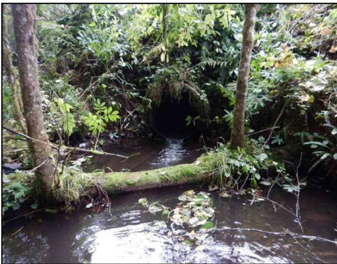
Figure 29. The old crossing was a 3 ft diameter concrete culvert that was a barrier due to slope.
