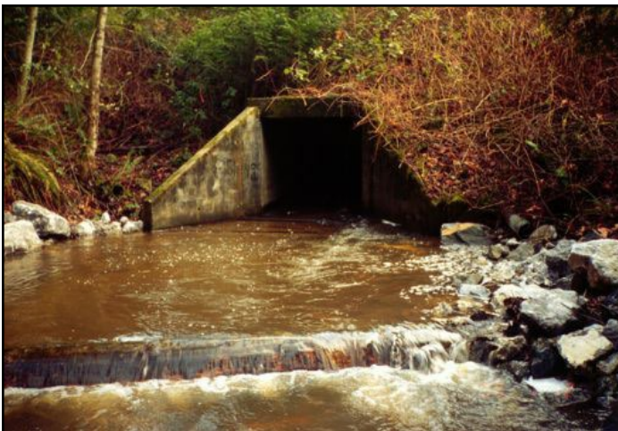
Figure 7. The old structure was undersized for the stream, a square concrete box 6 ft wide 6 ft tall and 120 ft long. The main issue for salmon was the water surface drop at the outlet which was too large for salmon to jump.
