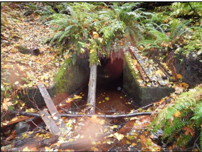
Figure 37. The old crossing was a 5 ft span by 4 ft rise concrete box culvert that was a barrier to fish passage due to velocity and depth.
