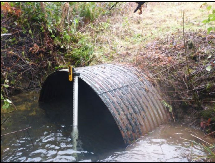
Figure 61. The old crossing was a box culvert extended with a 6 ft span by 3.6 ft rise squash, corrugated metal culvert that was a barrier due to lack of sufficient water depth during low flow.
