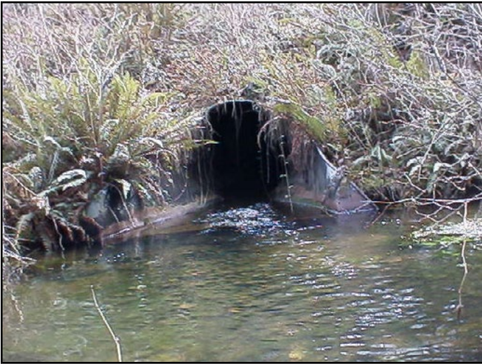
Figure 65. The old crossing consisted of a 4 ft square concrete box culvert cobbled to 4 ft round corrugated metal culvert extensions on either end. This undersized crossing was a barrier due to slope and a hydraulic drop at a joint where the metal culvert met the concrete culvert.
