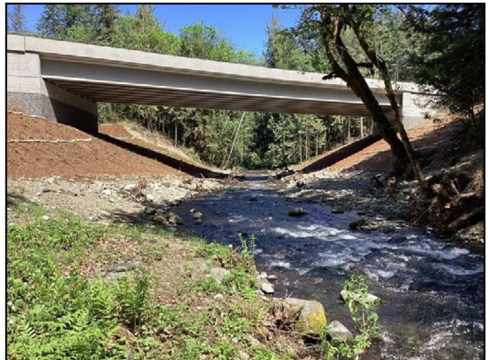
Figure 54. The new crossing is a 172 ft concrete girder bridge. The project was completed in February 2023 and adult salmon were observed spawning beneath of the new structure in September 2023.
