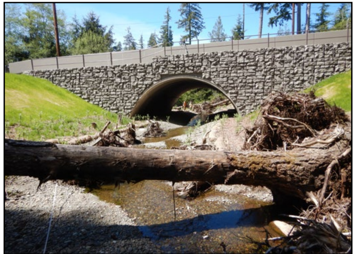
Figure 66. The new crossing is a 28 ft span by 15.6 ft rise structural plate, aluminum, bottomless arch.
