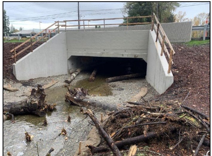
Figure 22. The new structure is a concrete bottomless arch culvert 23.6 ft span and 6.8 ft rise.
