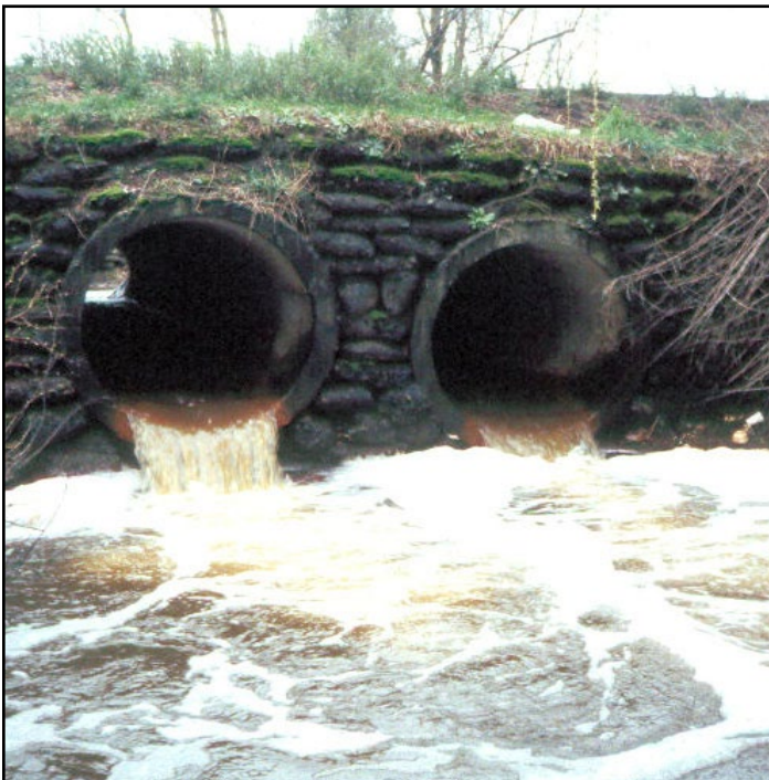
Figure 5. Two side-by-side 4 ft diameter concrete culverts. This site was a partial barrier due to hydraulic drop.
