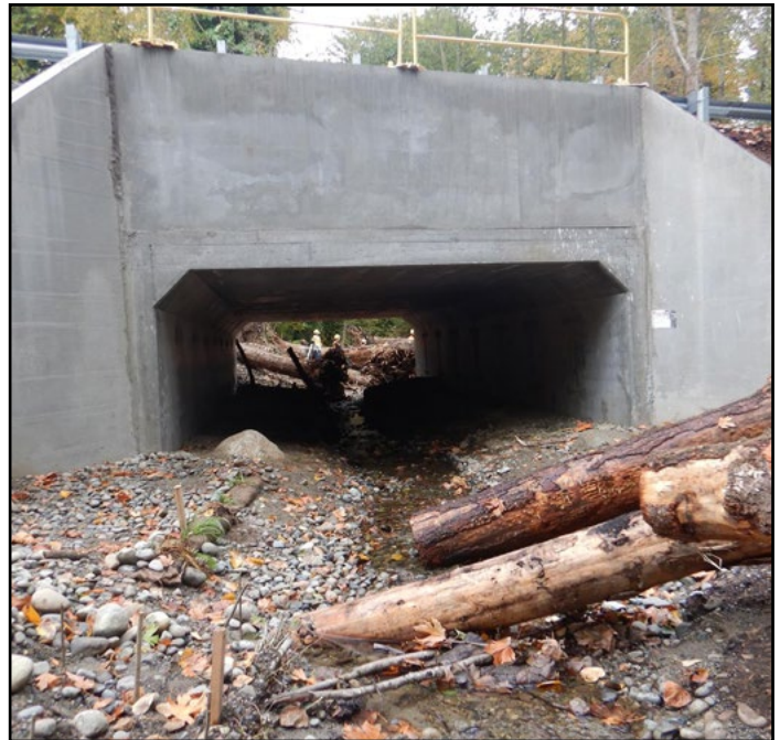
Figure 24. The new crossing is a 20 ft span by 12.6 ft rise concrete bottomless arch culvert.
