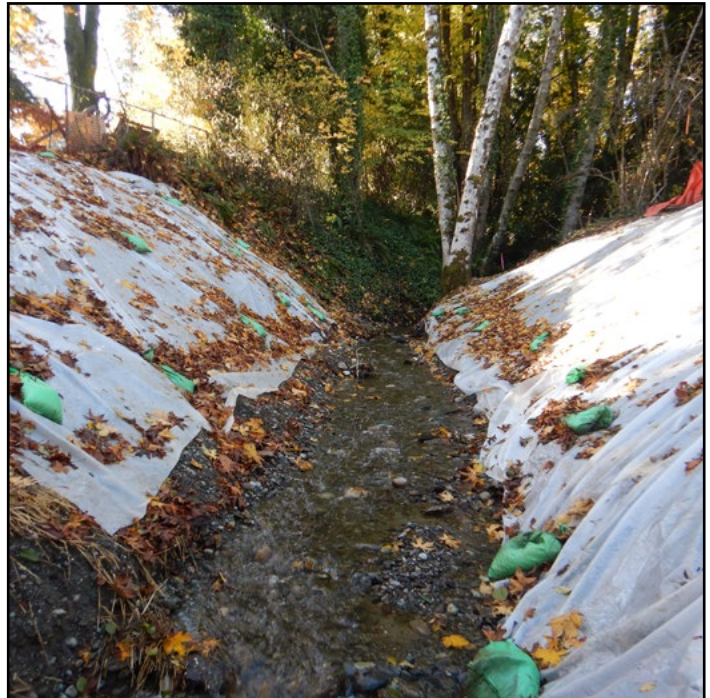
Figure 34. Structure-free open channel restores access to 0.18 miles of potential habitat for chum, coho, steelhead, coastal and resident cutthroat trout.
