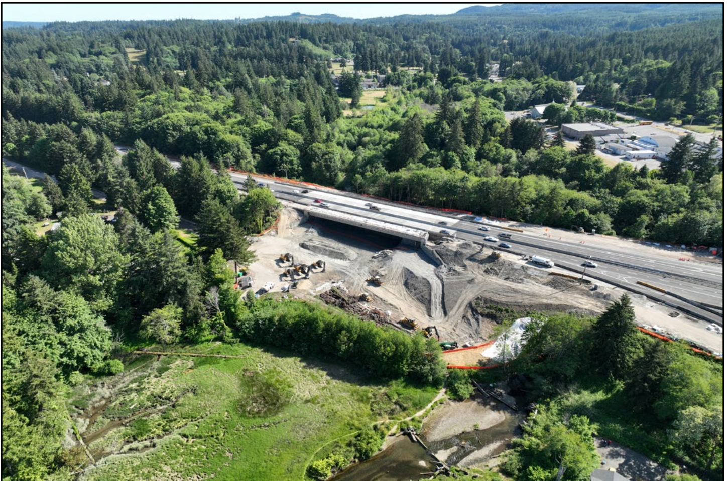
Figure 67. Chico Creek along SR 3, which is currently under construction, has been one of WSDOT's largest fish passage projects to date. This project has required extensive coordination across the watershed and involved the contributions of many groups, including tribes, the Recreation and Conservation Office, and other agencies like WDFW, the U.S. Navy, and Kitsap County. Being the most downstream barrier in an estuary and intertidal system, this correction will invite immediate benefits to fish and other species.
