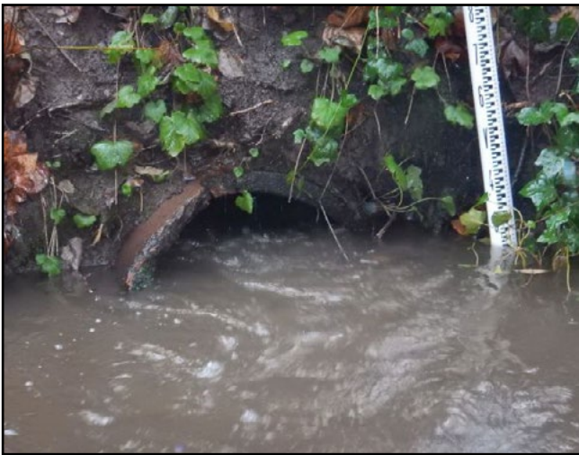
Figure 23. The old structure was a 2.0 ft diameter mixed material culvert. The downstream end was ceramic connected by a collection box to the upstream end, which was concrete.
