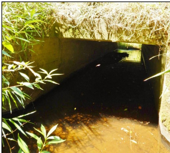
Figure 46. The old crossing was a 2-cell concrete box culvert with each cell measuring 5 ft span by 4 ft rise. The site was a barrier due to velocity.
