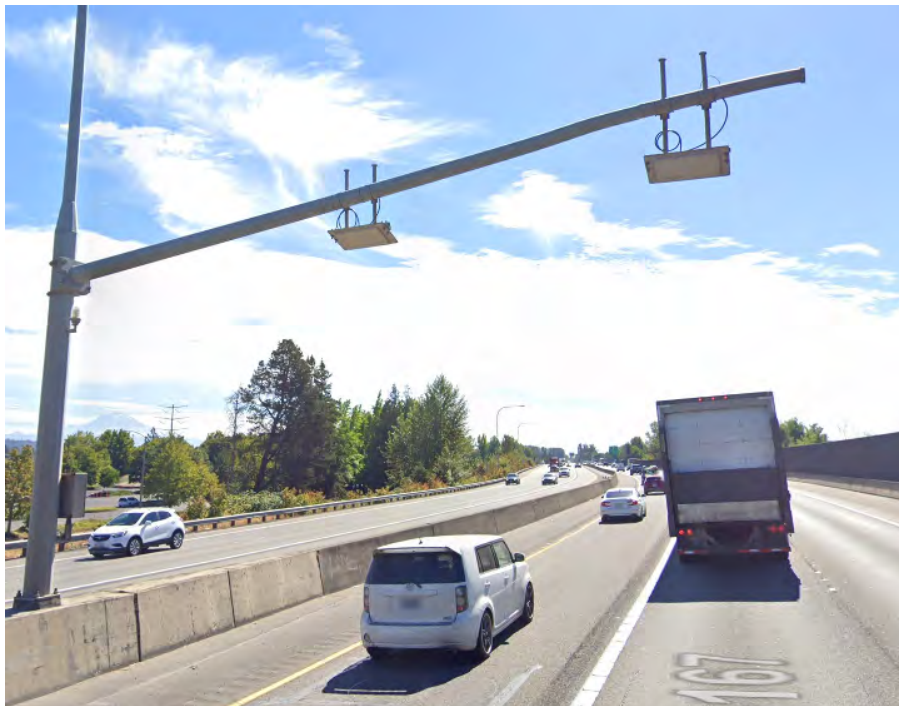
Figure 2. SR 167 Toll Collection Equipment
