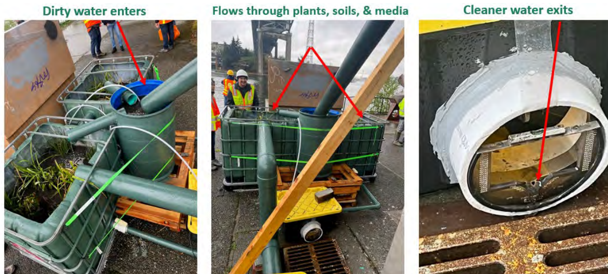
Adopt-a-downspout stormwater treatment test project.
