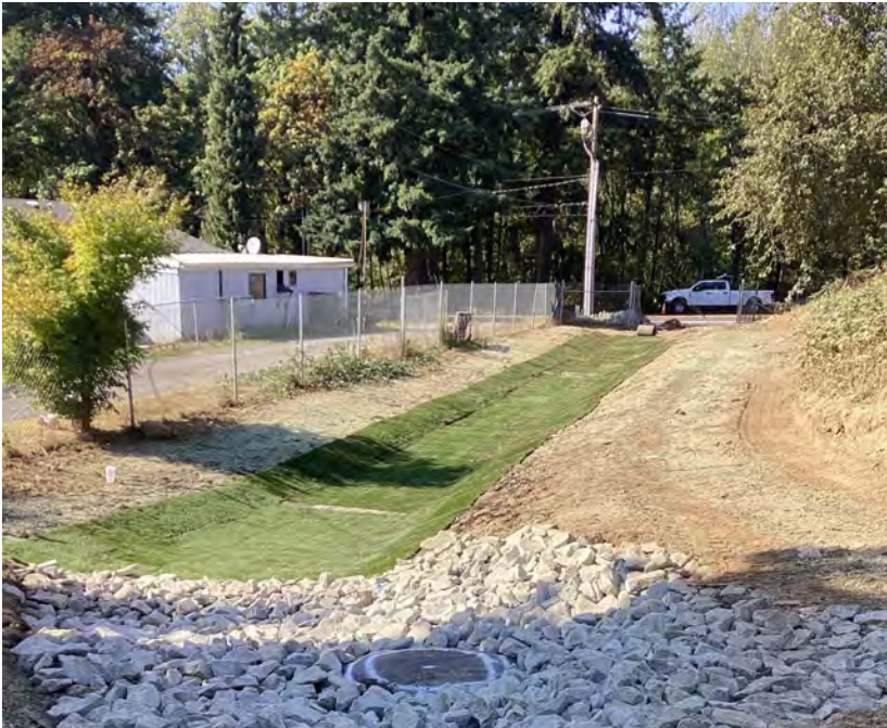
Figure 5. A bioswale near Salmon Creek is reconstructed by Southwest Region Area 1 crews.
