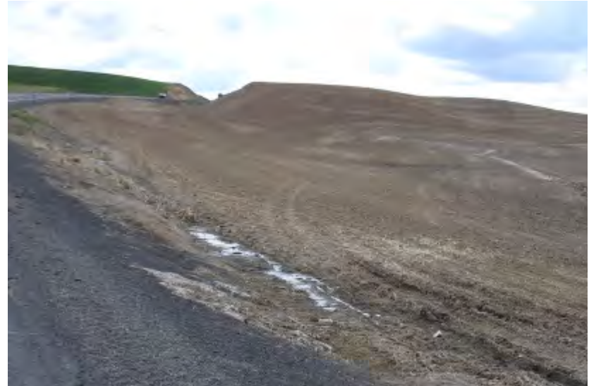
Figure 2. WSDOT works with Ecology to identify priority locations for remedying erosion problems associated with farming activity in some eastern Washington watersheds. Chronic erosion from farming activity is an ongoing maintenance and water quality challenge, as seen at this location on SR 27 within the Hangman TMDL.
