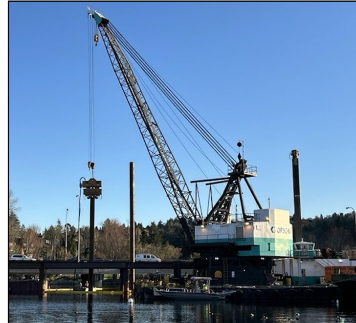
Crews use a vibratory hammer to drive piles near the Montlake lid.
