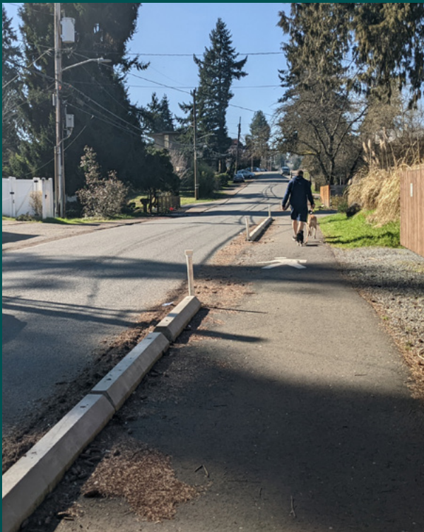
FIGURE 16 A low-cost walkway protected with precast concrete barriers in Seattle, WA.
